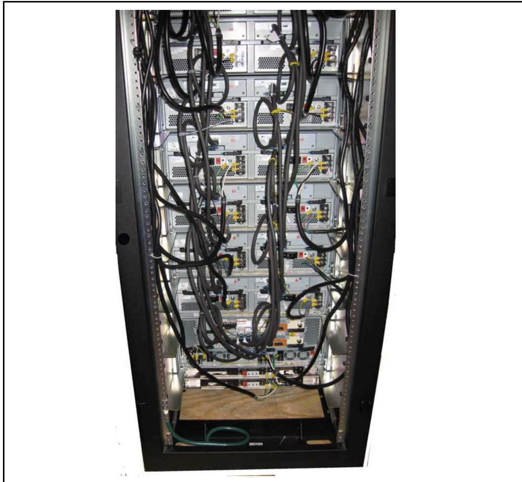
Figure 6-2: Seismic Rack - Rear View
